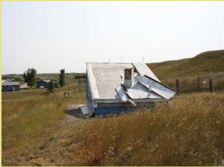
Bear Creek damage - typical
