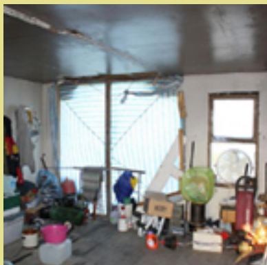
Interior damage – no electric or water
