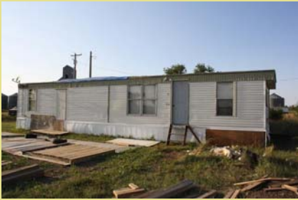
Damaged roof caused floors to warp Trailer still occupied
