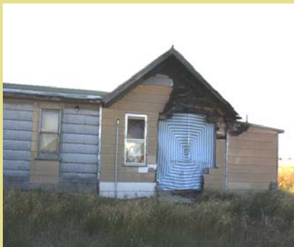
Indian Reservation Fire damaged home – still occupied!
