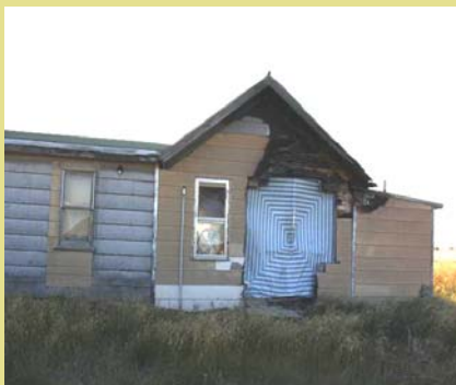
Indian Reservation Fire damaged home – still occupied!
